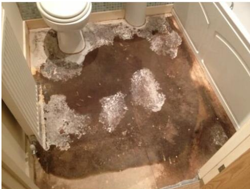
Wet floors leading to failure of chipboard
