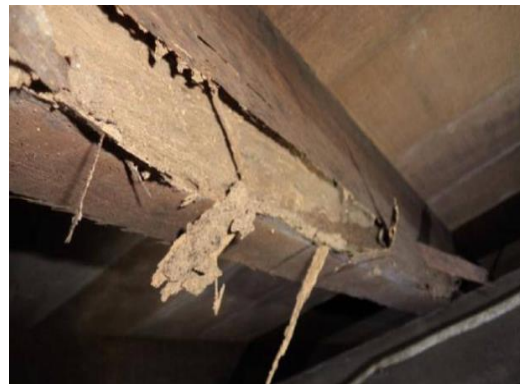
Borer or moisture causing failure in floor joists
