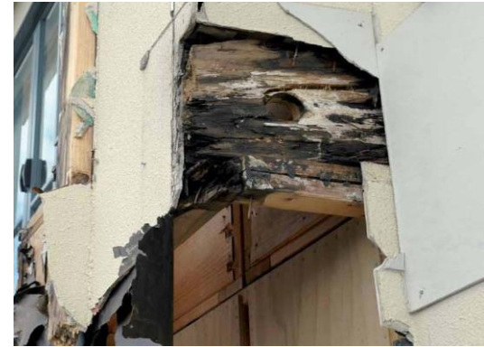
Watertight issues (leaky homes)
