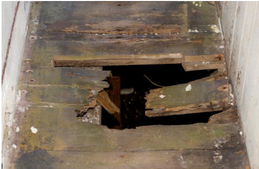
Damage to floorboards
